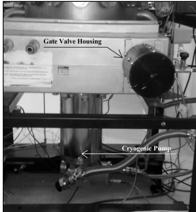
Figure 76: Cryogenic Pump and Gate Valve
